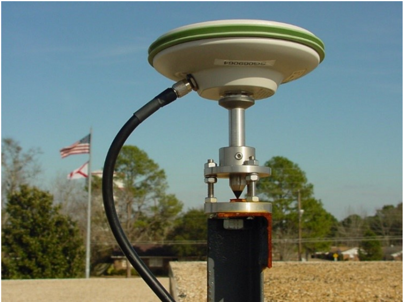
Figure 8. A CORS antenna mounted to a post. Source: National Geodetic Survey .
